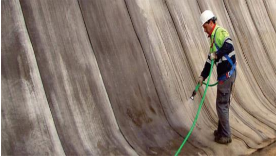
Figure 2.2.5: Spray The Fiber Surface with Water Until It Feels Wet to Touch for Several Minutes After Spraying.
