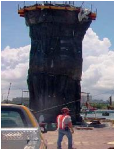
Fig. 3. A bridge column uses surface insulation to minimize the temperature difference between the interior and the surface
