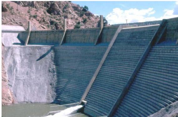
Fig. 9. RCC dam of Santa Cruz River in Argentina popularly known as Puerto Santa Cruz Dam
