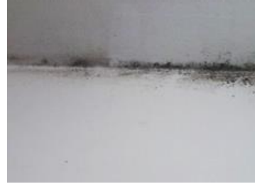
Fig. 2. Photo of mold in the junction area of the exterior wall and attic floor surface
